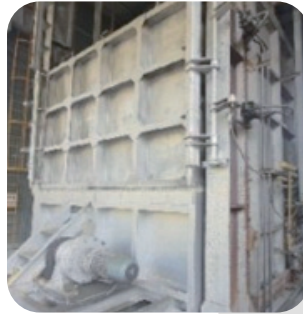
Heat treating furnace
